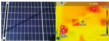
Fig. 1 Shading and hotspots caused by lightning rod 1
